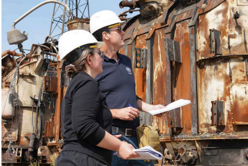
The first IAEA Ukraine mission to electrical substations took place on September 12. Photo: NAEK Energoatom
